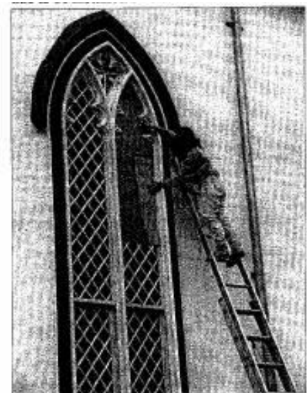
Susan Frocheur-Jernejcic fine-tuning a template to be used for patterning the new protective glazing system.
